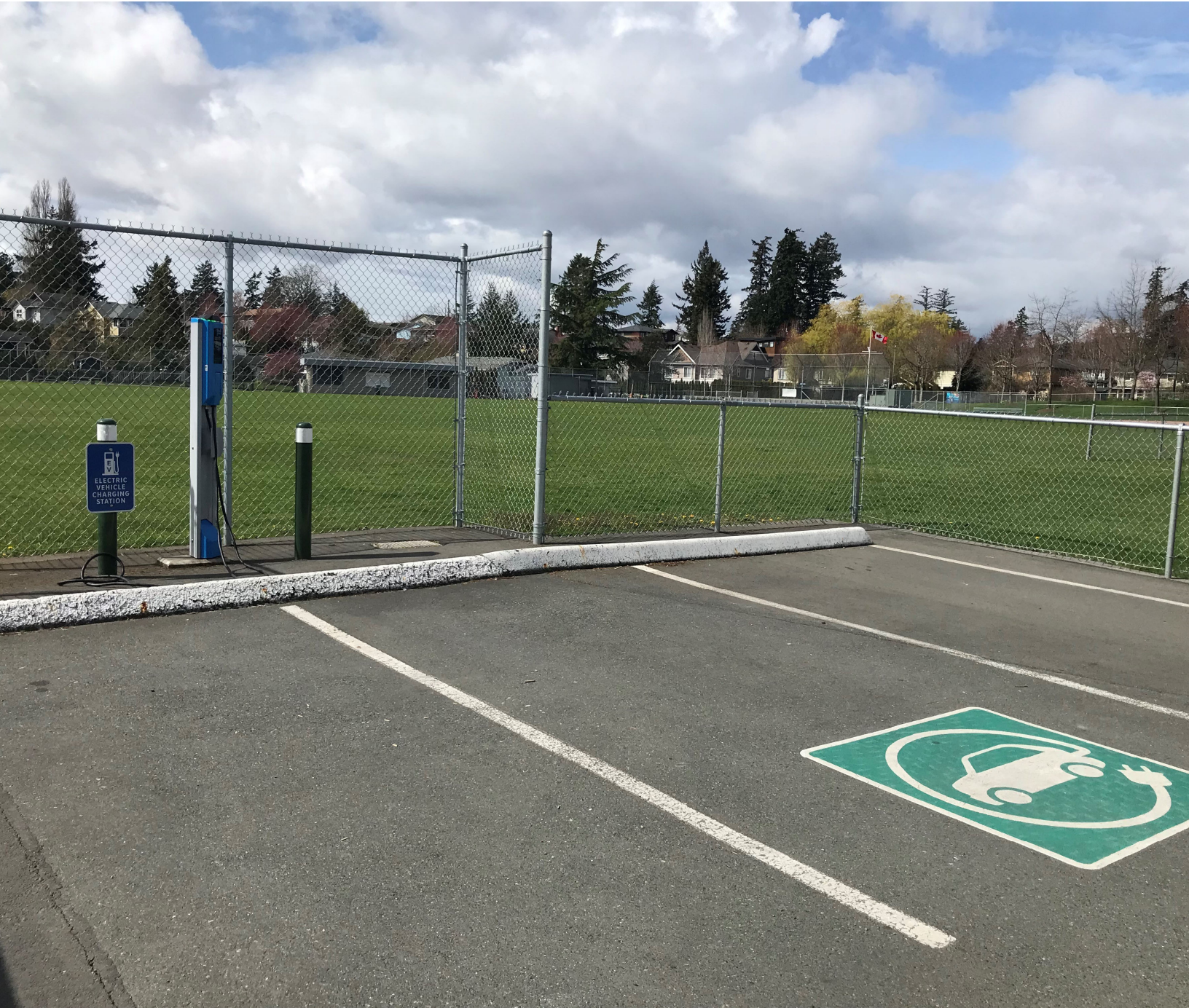
Charging Station at Helmcken Centennial Park
